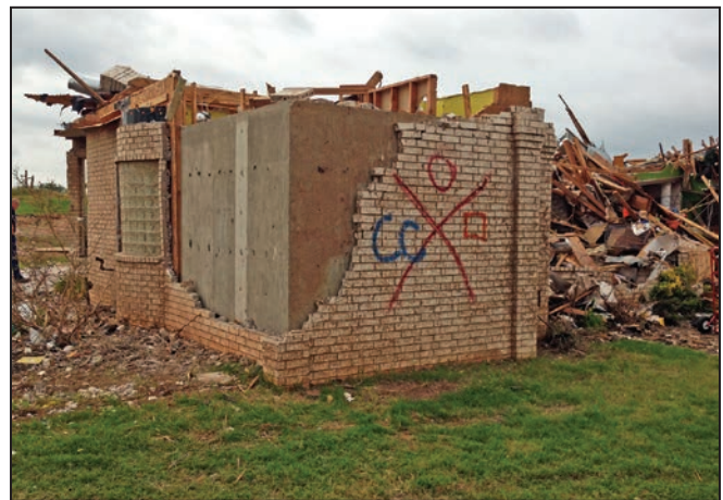
Figure 5-2: Site-built safe room that withstood the impact of the Moore tornado (Moore, OK, 2013)
